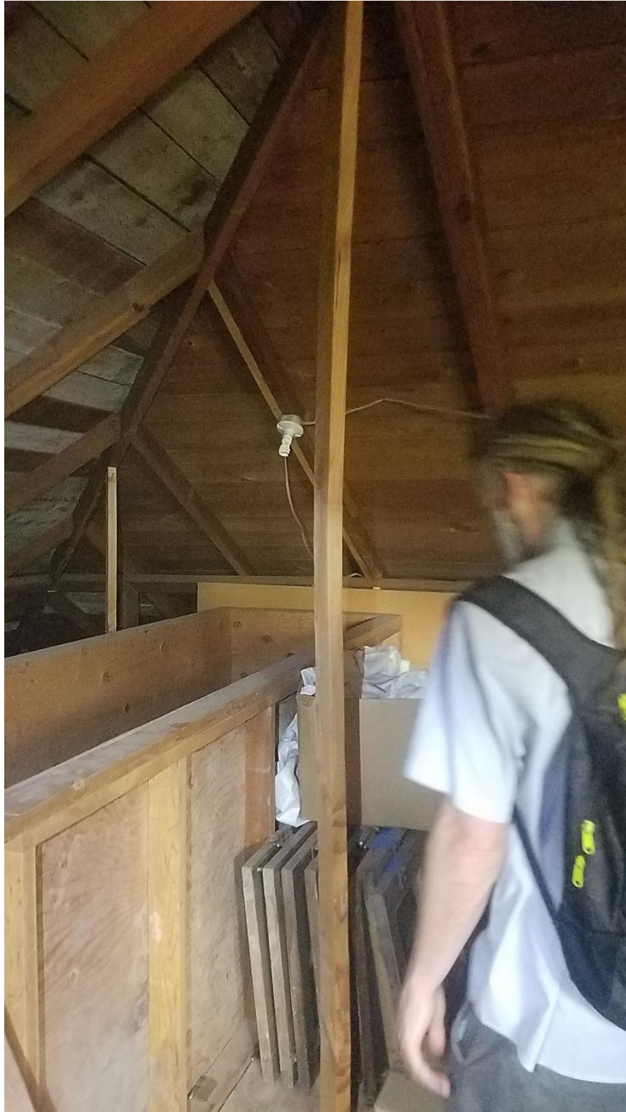
Figure 3. Winburn Way Community Center, Over-stressed hip support
