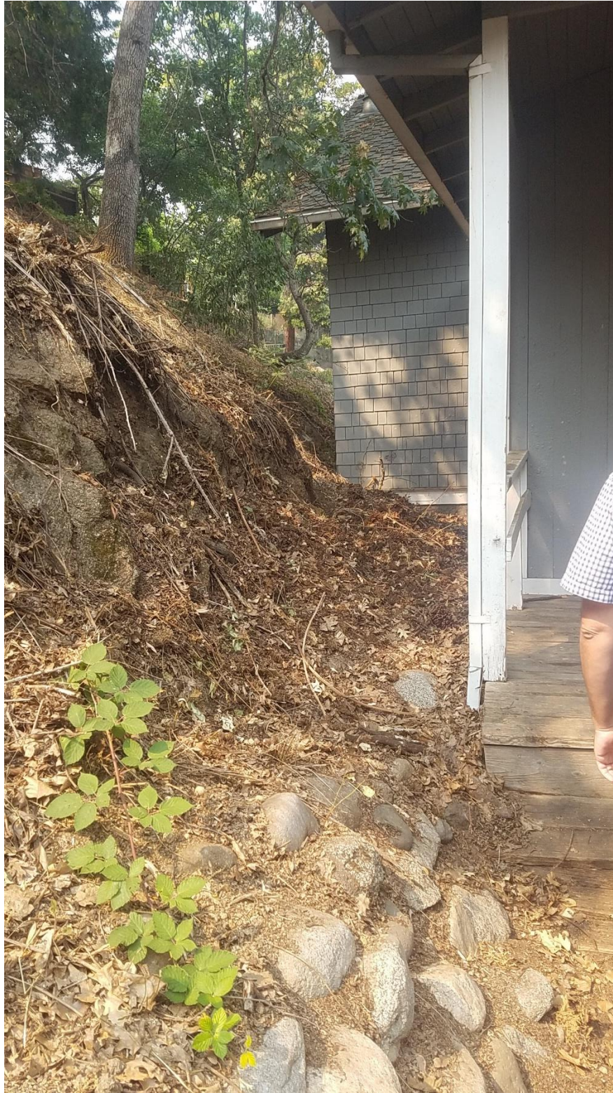
Figure 4. Winburn Way Community Center, Rear Sloughing Conditions
