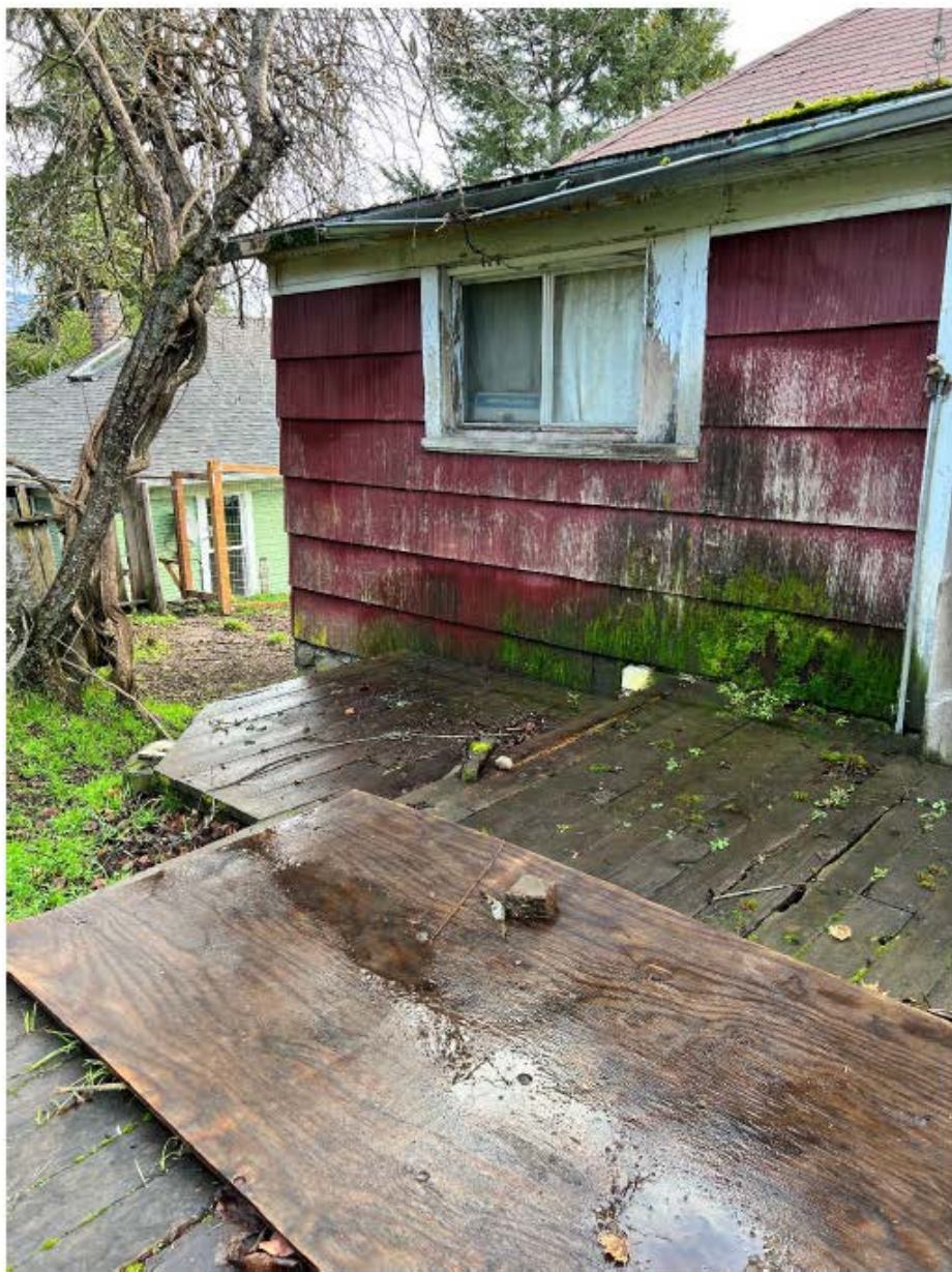
Figure 7: West wall. Substantial rotted wall with raised spigot to right
