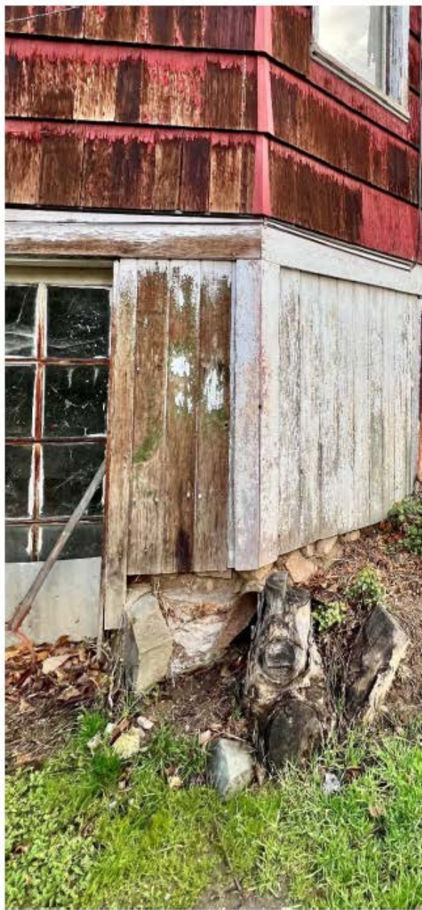
Figure 3: Long dead tree protruding from the foundation.
