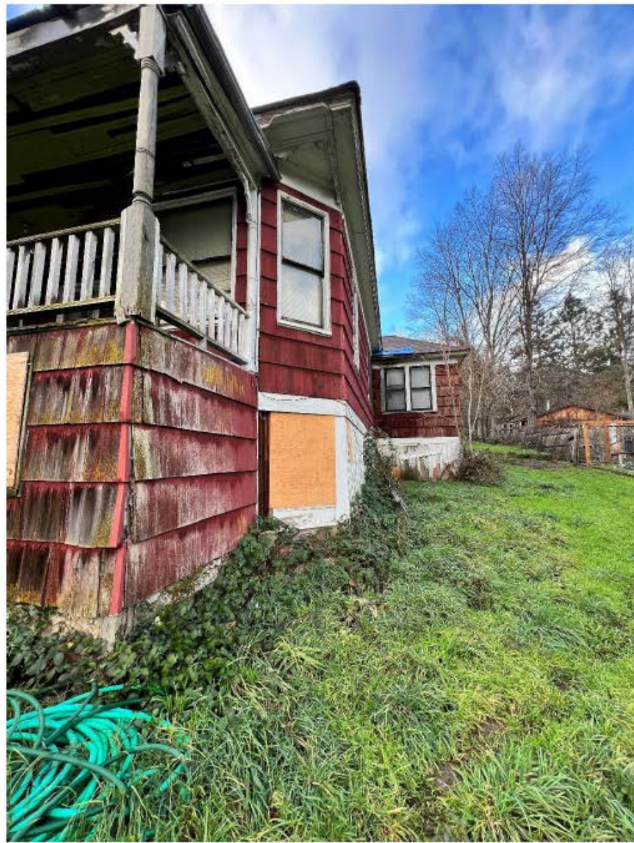
Figure 8: North Wall and northwest corner. Porch post cracked, off of the corner. Failing roof evident with blue tarp at roof valley. Valley patched significantly, the wall under tarp is black with rot and mold
