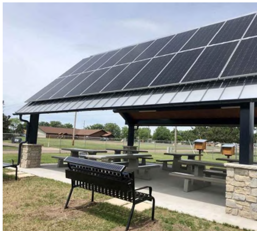
SOLAR PANELS ON SHADE STRUCTURE ROOF
