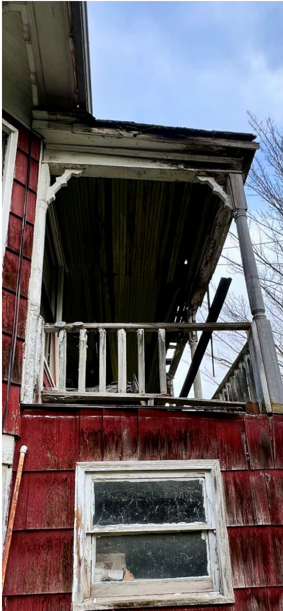
Figure 1: Front porch - daylight coming through roof, rotten fascia
