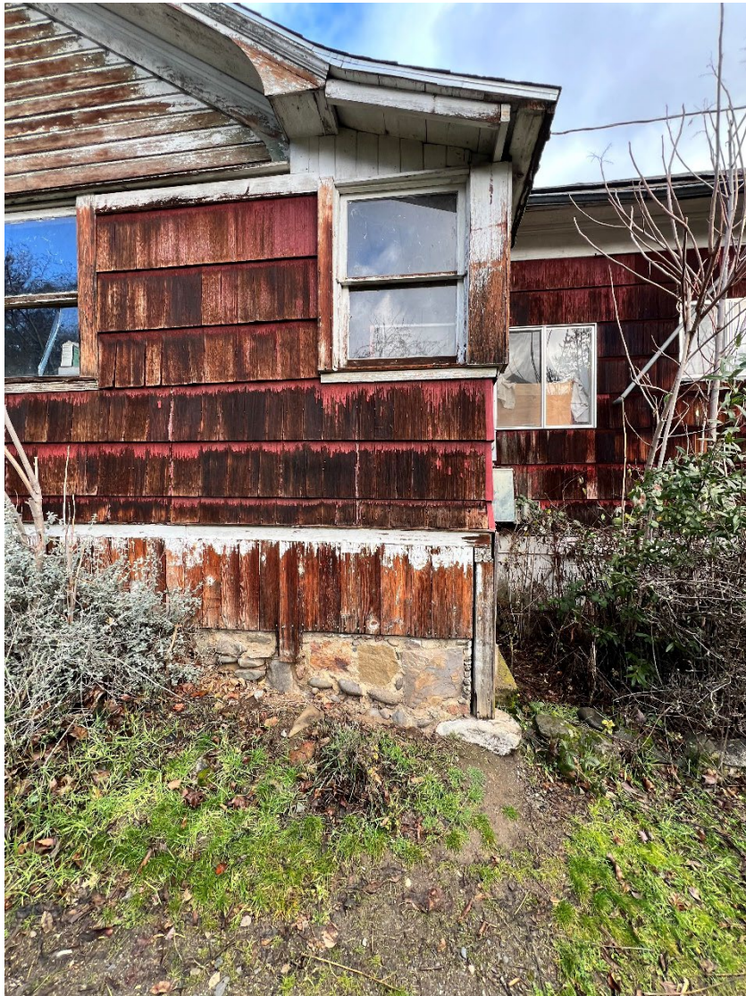
Figure 5: At SE corner of house facing driveway. Corner post shifting from the rim joist and the wall failure continues up to the top plate.
