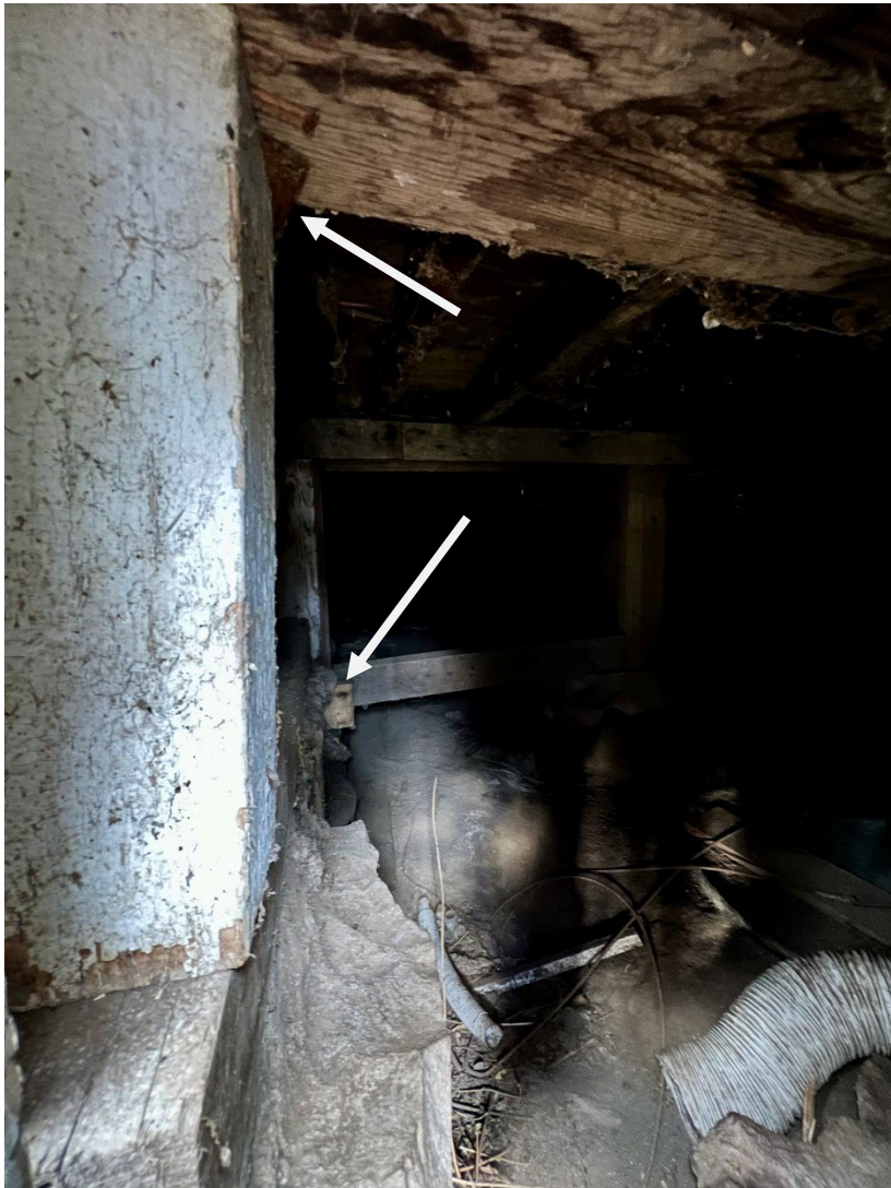
Figure 9: Crawlspace access on SE side. Wood blocks jammed between floor joist and stemwall posts.
