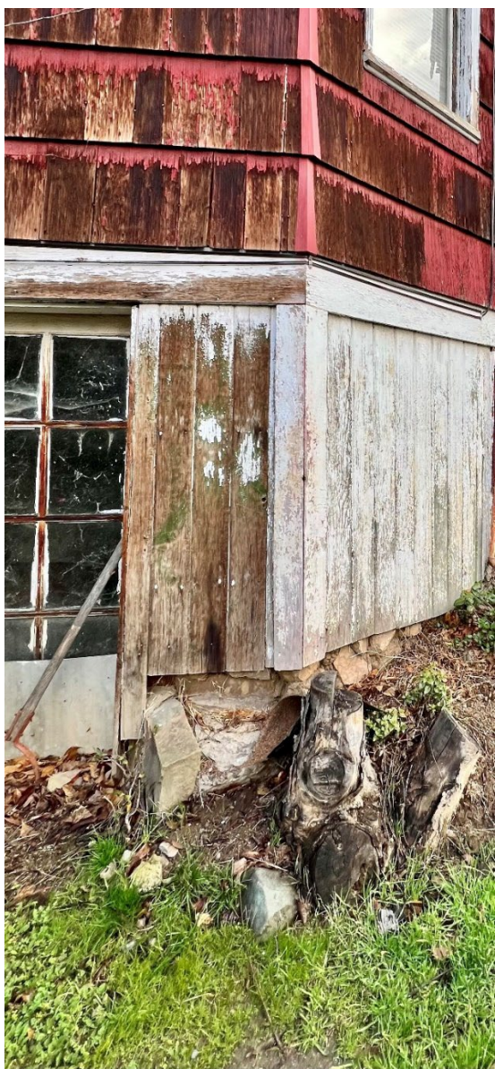
Figure 3: Long dead tree protruding from the foundation.
