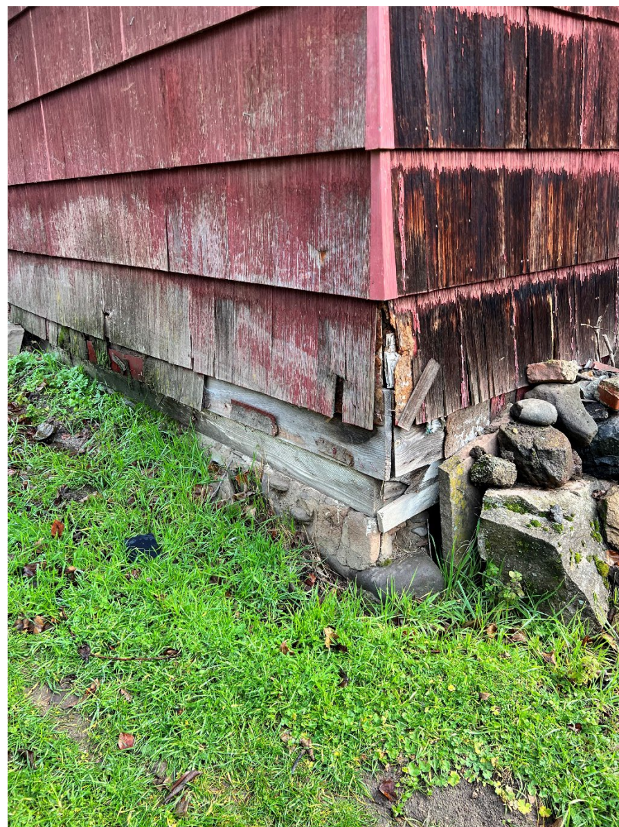
Figure 4: SE corner of foundation shows substantial crack in the corner stone which sits upon a round rock
