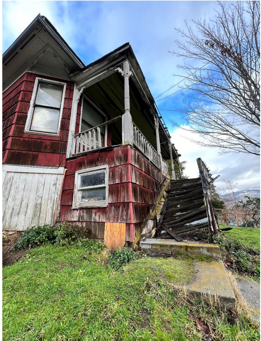
Figure 2: Front steps to front porch and front entry. Window opening showing damage where evidence of foundation failure below. Wall is buckling to left of window.
