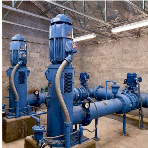
1 of 2 (50 hp) pumps proposed for replacement
