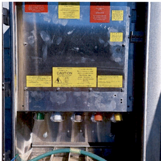
BPS generator electrical power inlet cabinet
