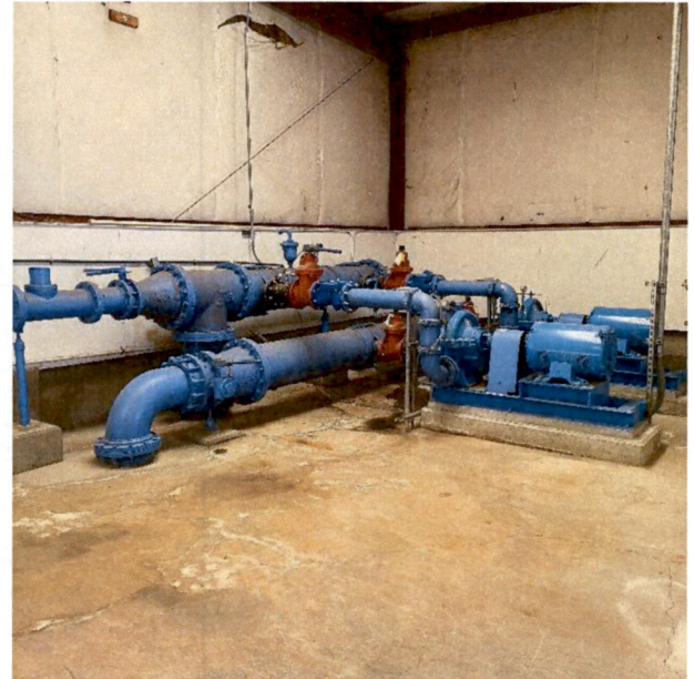
Existing pumps inside the Talent BPS
