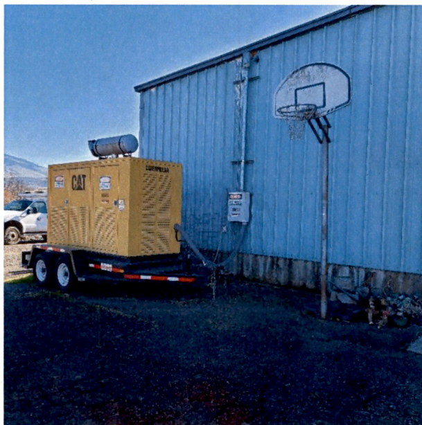
Existing generator at the Talent BPS
