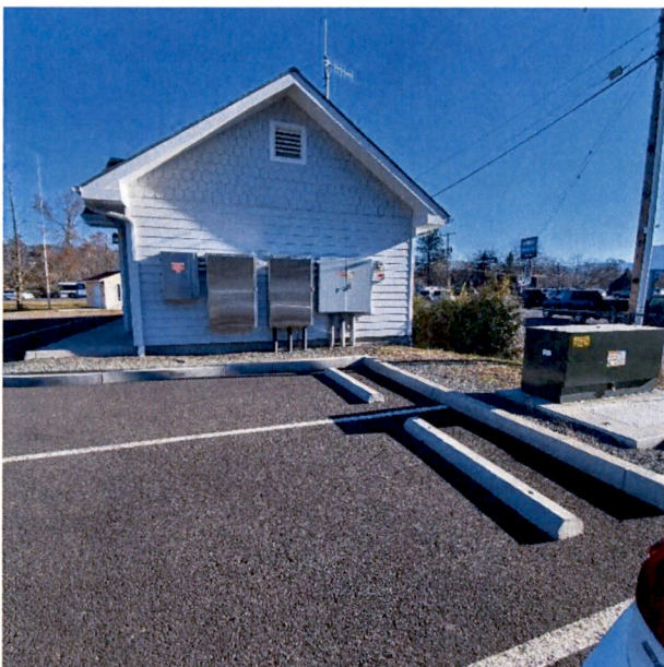
Ashland BPS proposed new generator location
