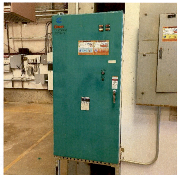
Existing automatic transfer switch in Talent BPS
