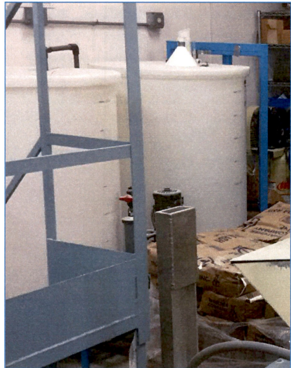
Photo 3-12 – Filter Polymer Aid Feed Tanks
