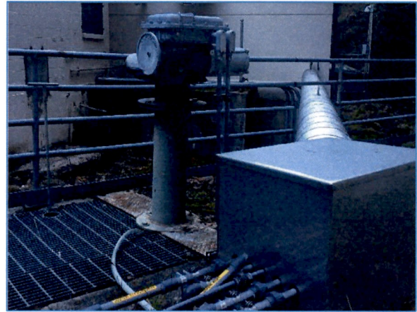
Photo 3-4 – Influent 36-inch Butterfly Valve
