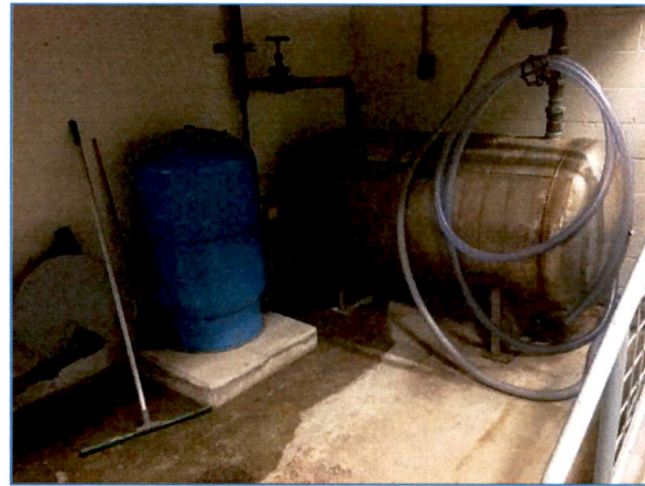
Photo 3-2 – Potable Water Storage Tank and Hydro-Pneumatic Tank
