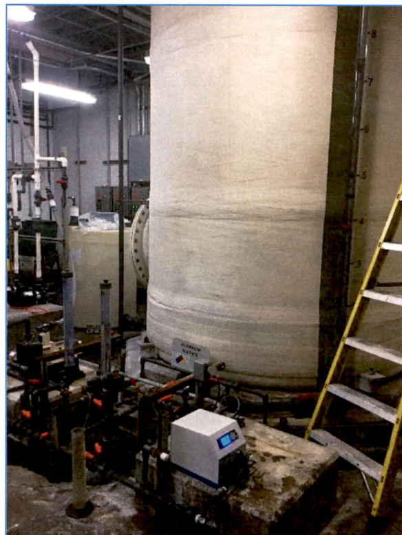
Photo 3-7 – Base and Pedestal of Alum Tank
