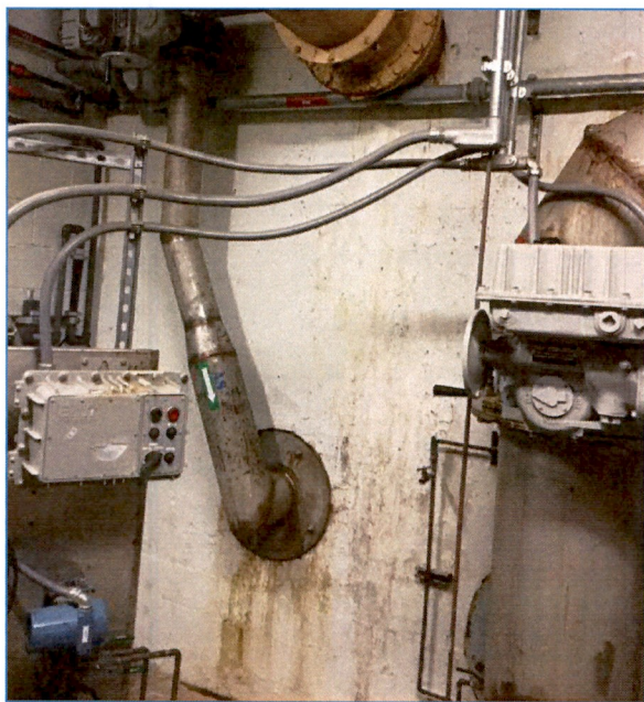
Photo 3-20 – Air Scour Air Supply (Evident Leakage)
