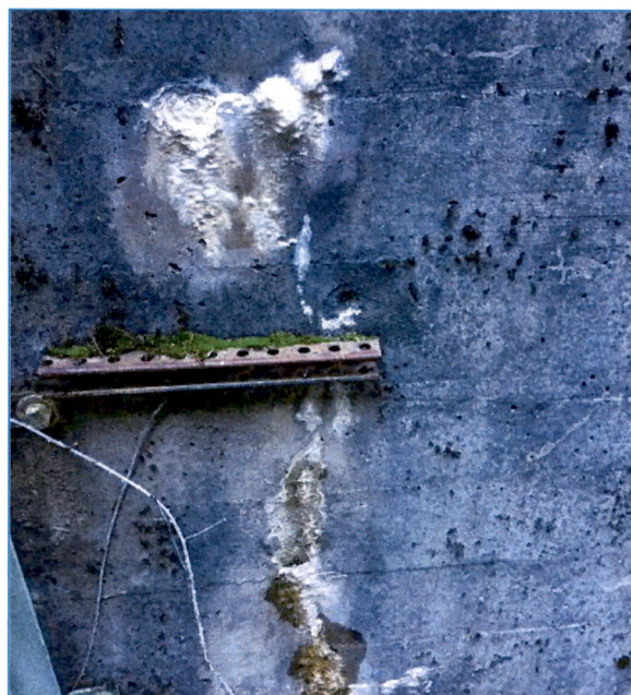
Photo 3-21 – Efflorescence on Exterior Dual Media Filter Wall
