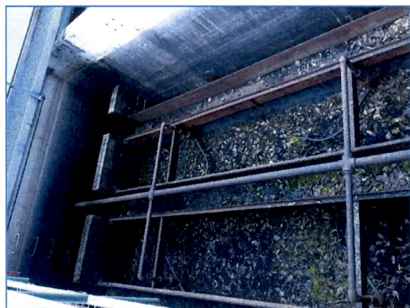
Photo 3-19 – Abandoned Dual Media Filter #7
