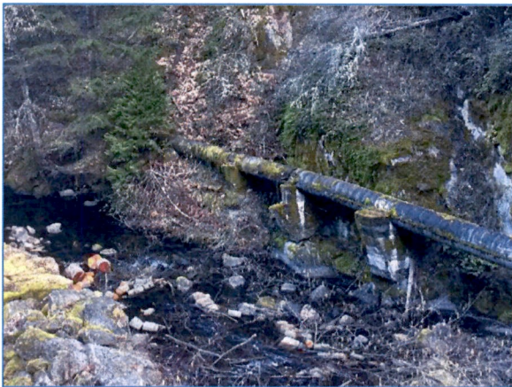
Photo 3-5 – Talent Irrigation District Influent Pipeline
