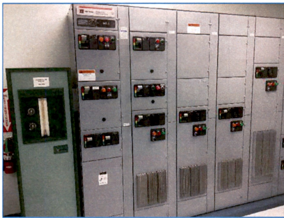
Photo 3-22 – Motor Control Center
