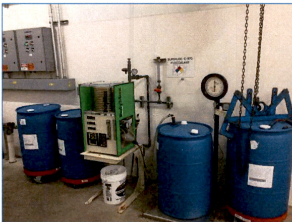
Photo 3-13 – Cationic Polymer Feeder
