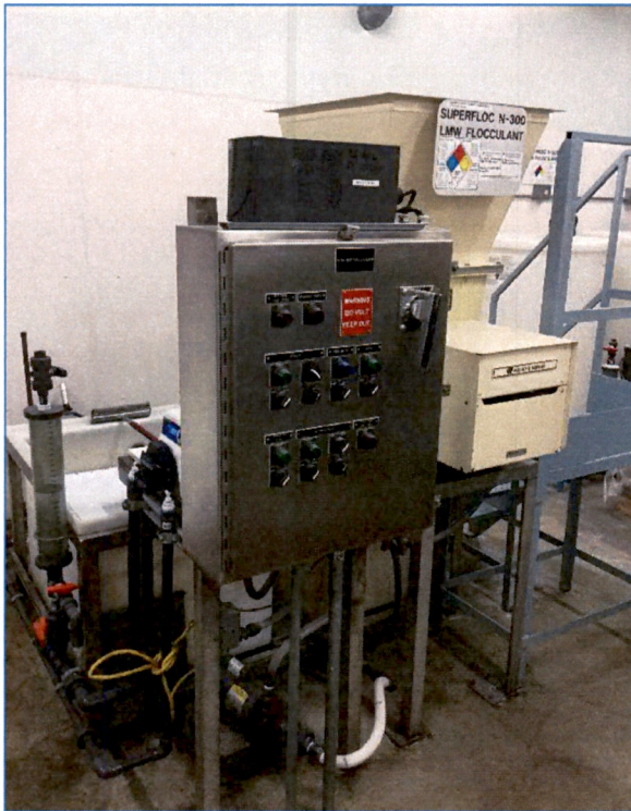
Photo 3-11 – Filter Polymer Aid Hopper and Mixing Tank
