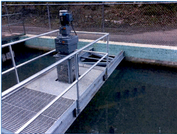
Photo 3-16 – Flocculation Basin and Paddle Mixer
