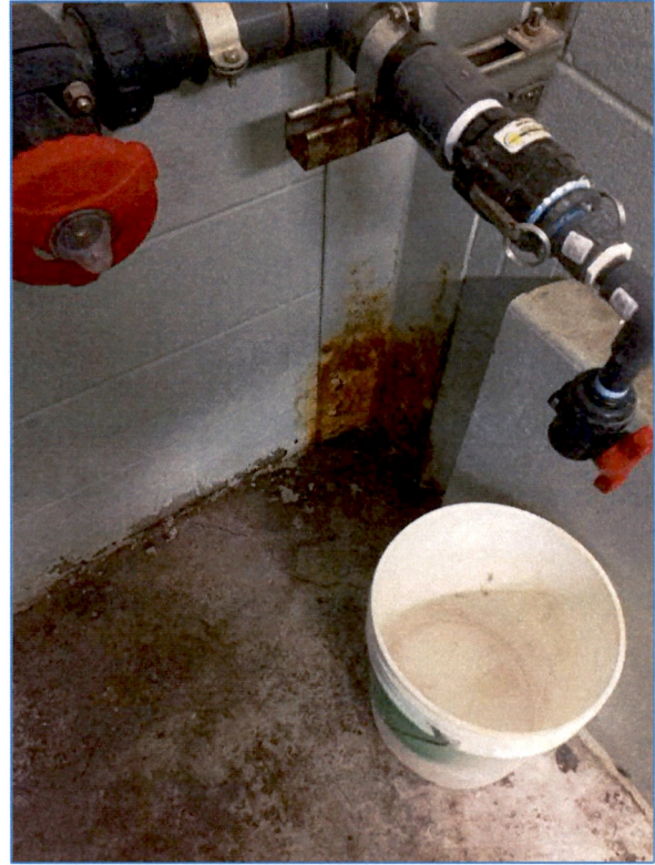
Photo 3-15 – Corrosion in Chlorine Building
