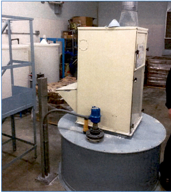
Photo 3-8 – Soda Ash Hopper
