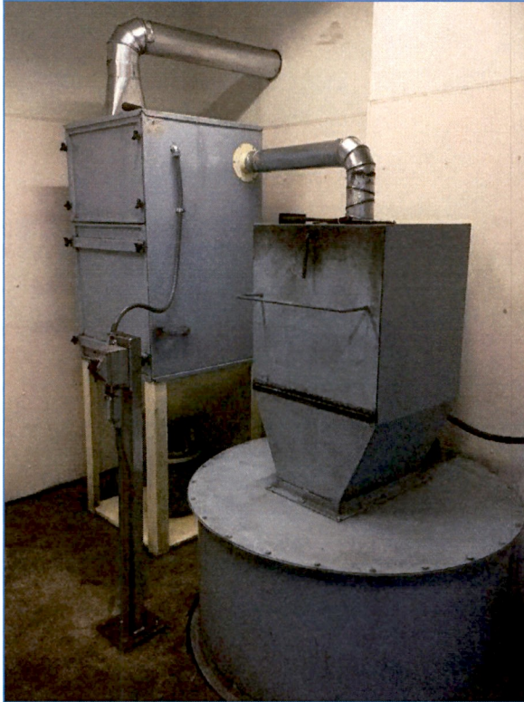
Photo 3-10 – Powdered Activated Carbon Hopper
