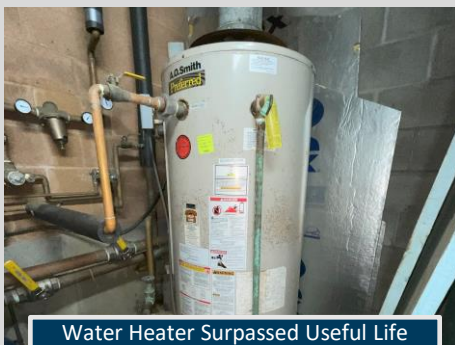
Water Heater Surpassed Useful Life Expectancy
