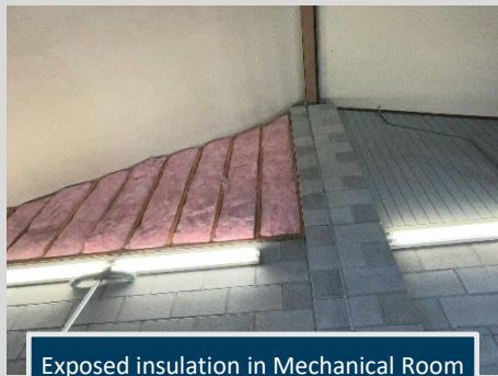
Exposed insulation in Mechanical Room
