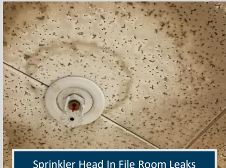
Sprinkler Head In File Room Leaks
