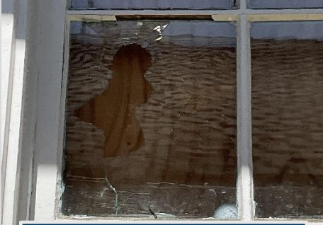
Single Pane Windows Damaged
