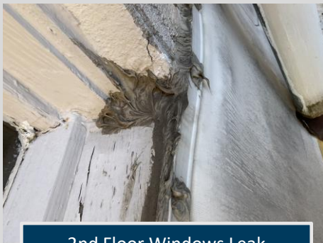
2nd Floor Windows Leak
