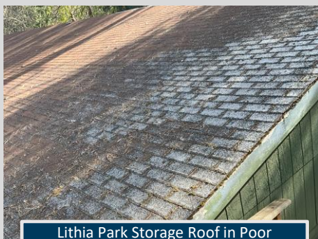
Lithia Park Storage Roof in Poor Condition
