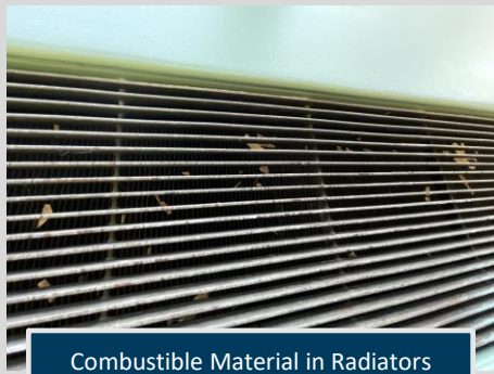
Combustible Material in Radiators
