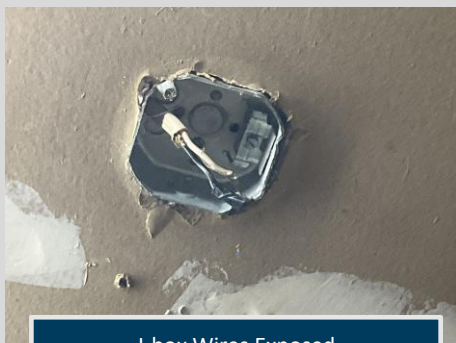
J-box Wires Exposed
