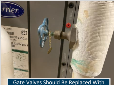
Gate Valves Should Be Replaced With Ball Valves
