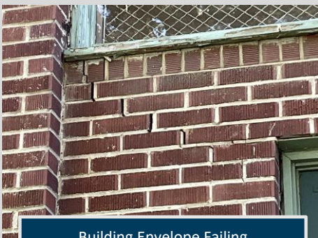
Building Envelope Failing
