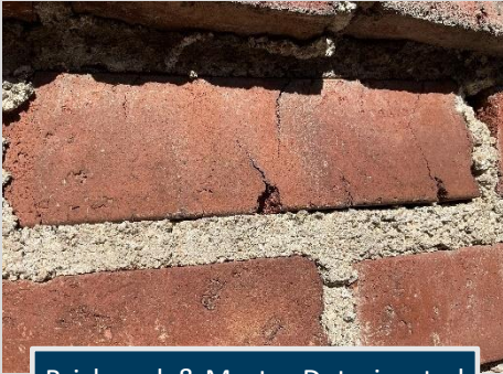
Brickwork & Mortar Deteriorated
