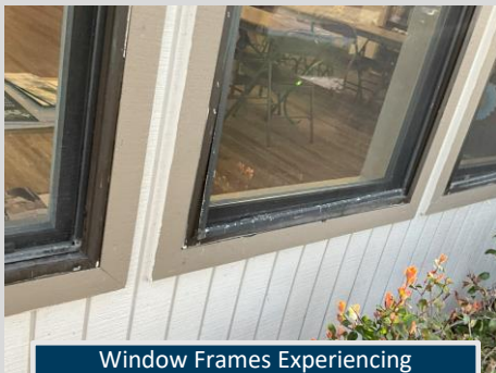
Window Frames Experiencing Weathering
