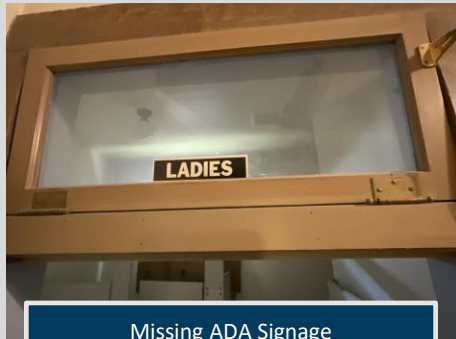
Missing ADA Signage
