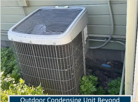
Outdoor Condensing Unit Beyond Industry Expected Life
