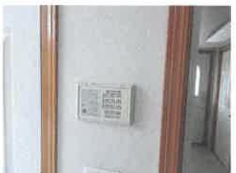
Heating and cooling ctrl.
