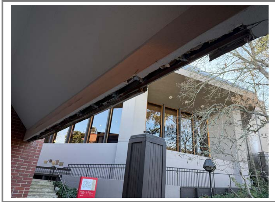
View of balcony covering with areas of deterioration
