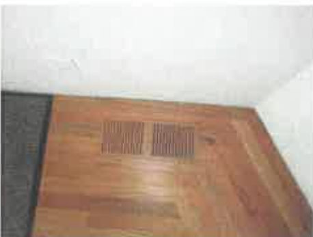
Heating register detail
