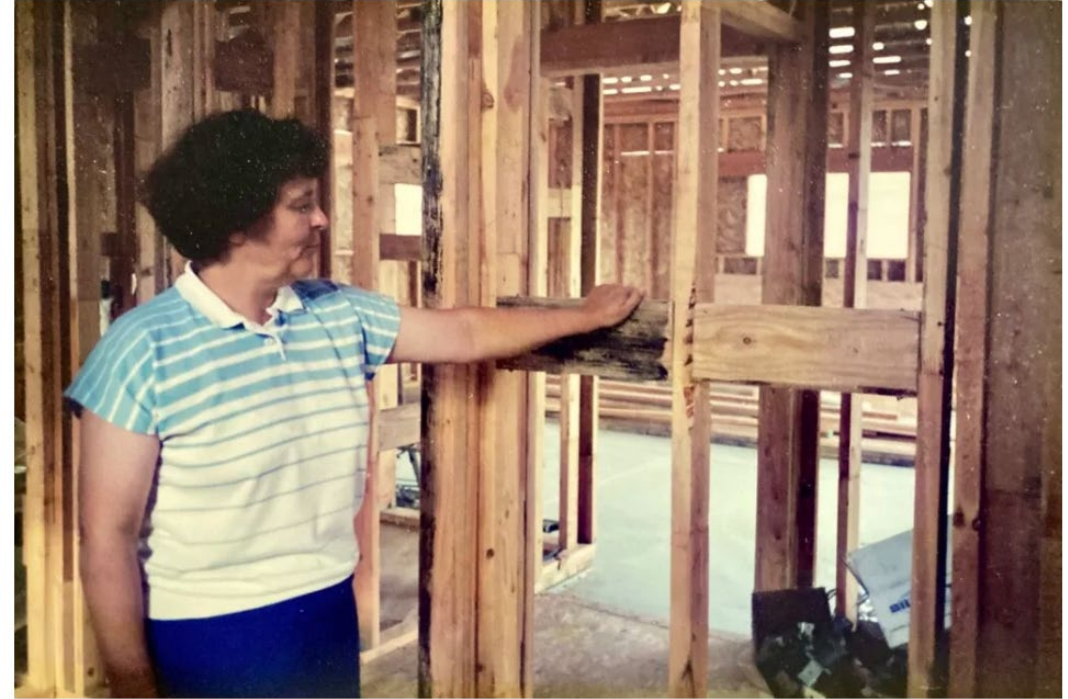
Madeline Hill in a future bathroom, showing where grab bars could be attached to wall when homeowner was ready. (photo by Hunter Hill, Madeline Hill collection, photo taken mid-1990s)
