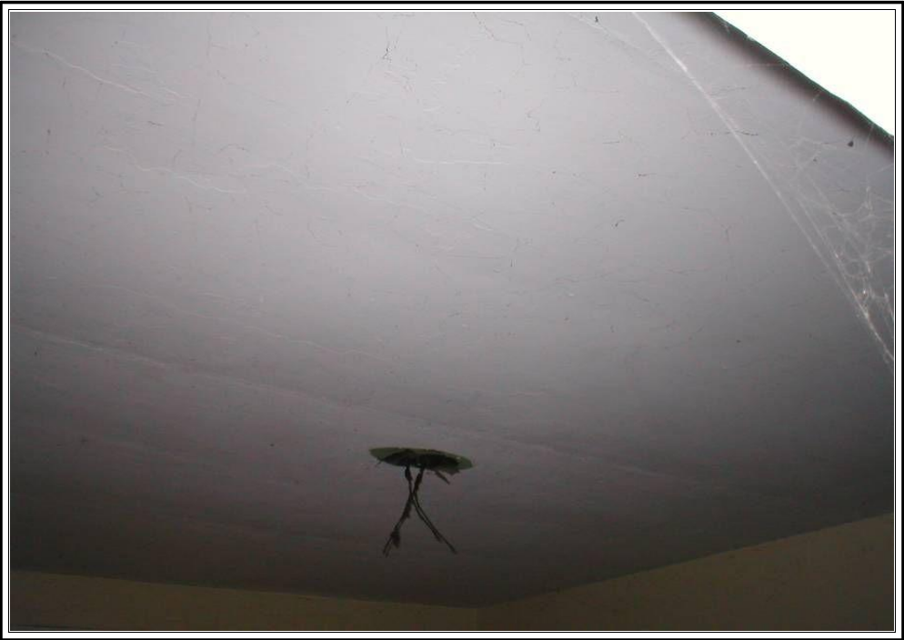
missing light fixture
