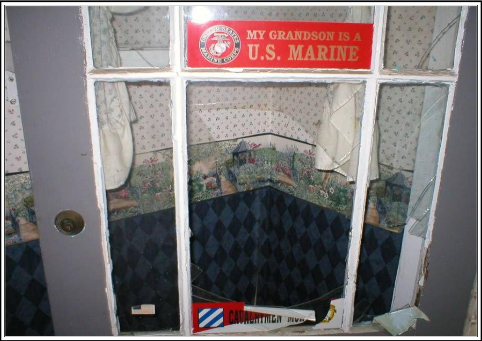
interior door (broken winow)
