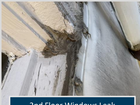
2nd Floor Windows Leak
