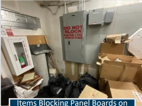
Items Blocking Panel Boards on 2nd Floor
