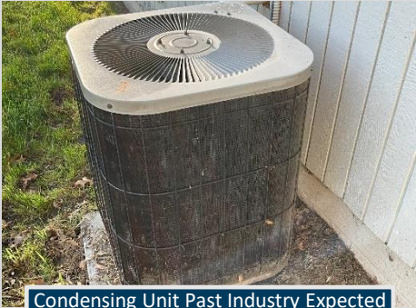
Condensing Unit Past Industry Expected Life
