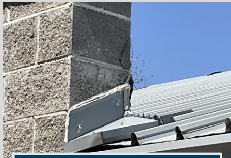
Flashing Needs Replacement
