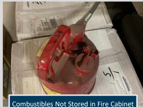
Combustibles Not Stored in Fire Cabinet
