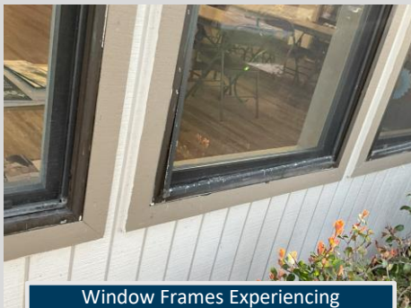
Window Frames Experiencing Weathering
