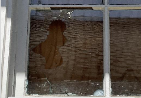
Single Pane Windows Damaged
