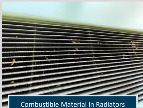
Combustible Material in Radiators
