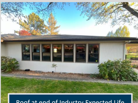
Roof at end of Industry Expected Life
