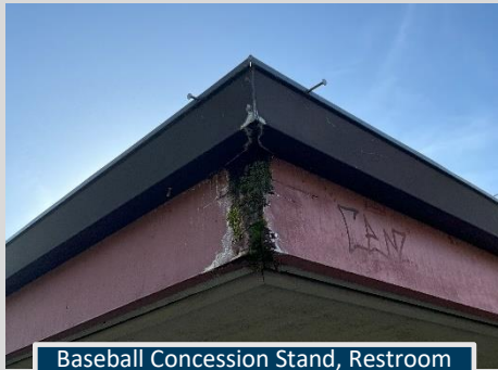
Baseball Concession Stand, Restroom and Clubhouse Roof Fascia Rotting
