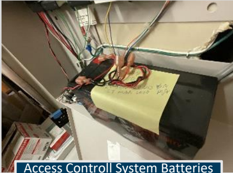
Access Control System Batteries Should be Replaced.
