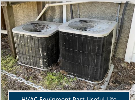
HVAC Equipment Past Useful Life
