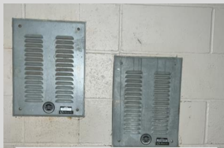
Softball Concession Stand, Restroom and Clubhouse Unit Heaters Exceeding Useful Life
