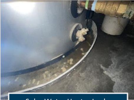
Solar Water Heater Leaks
