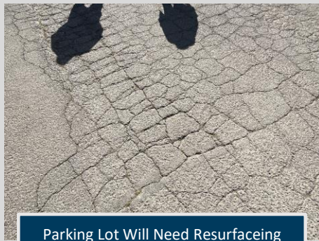
Parking Lot Will Need Resurfacing
