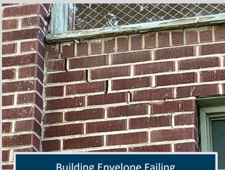
Building Envelope Failing
