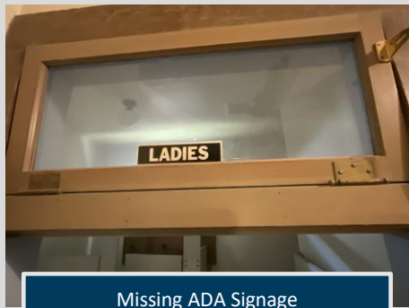
Missing ADA Signage
