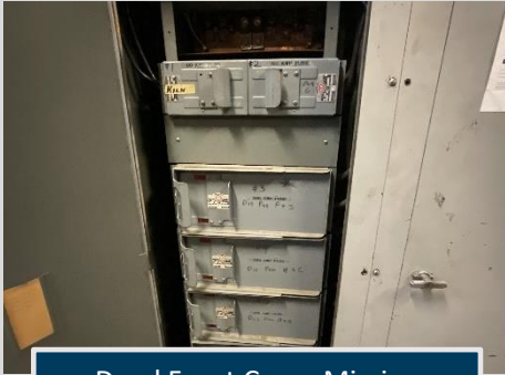
Dead Front Cover Missing
