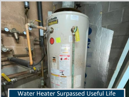
Water Heater Surpassed Useful Life Expectancy
