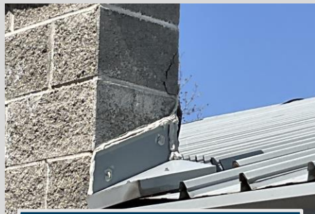
Flashing Needs Replacement
