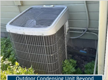
Outdoor Condensing Unit Beyond Industry Expected Life
