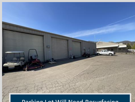
Parking Lot Will Need Resurfacing
