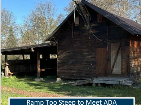
Ramp Too Steep to Meet ADA Requirements
