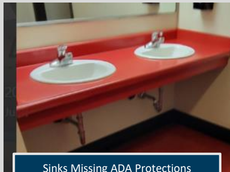
Sinks Missing ADA Protections
