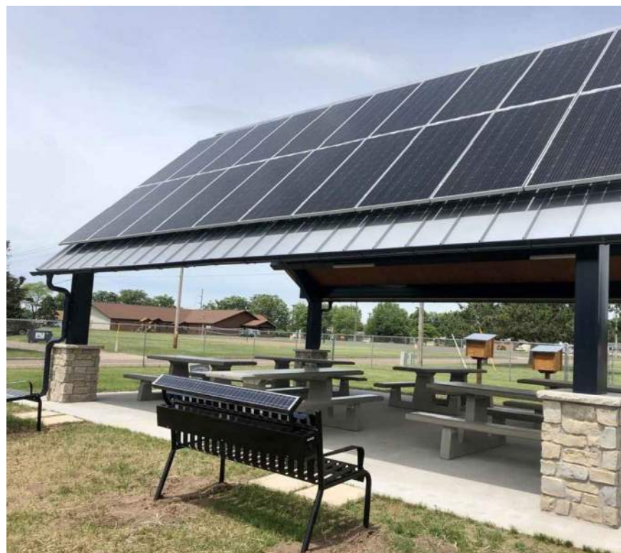
SOLAR PANELS ON SHADE STRUCTURE ROOF
