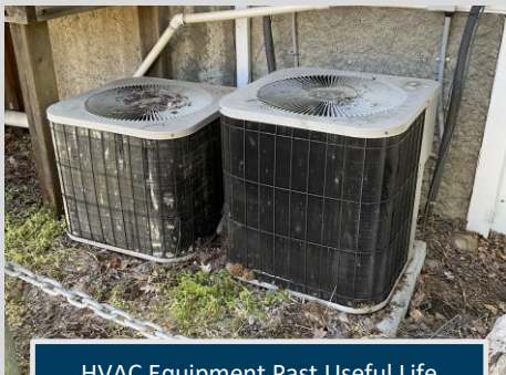
HVAC Equipment Past Useful Life
