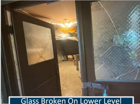
Glass Broken On Lower Level Storefront Exterior Doors
