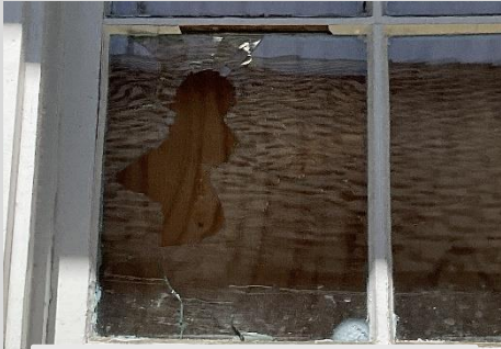
Single Pane Windows Damaged
