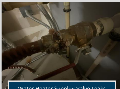
Water Heater Supply Valve Leaks
