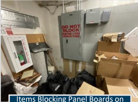
Items Blocking Panel Boards on 2nd Floor
