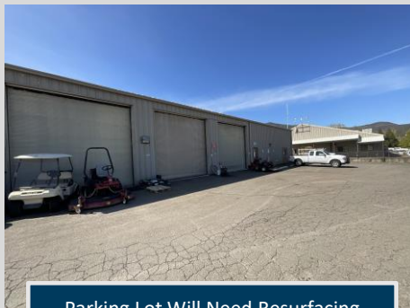
Parking Lot Will Need Resurfacing
