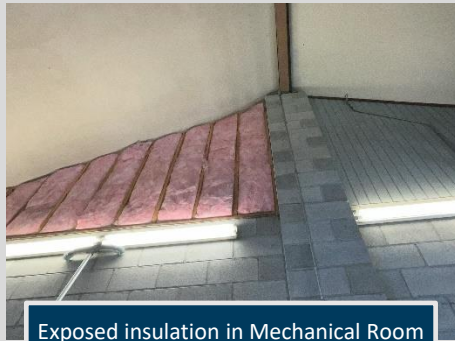
Exposed insulation in Mechanical Room
