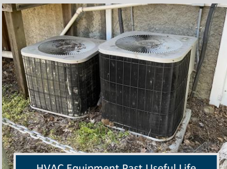
HVAC Equipment Past Useful Life
