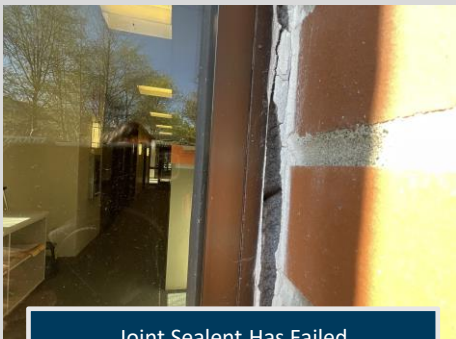
Joint Sealant Has Failed
