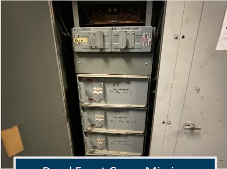
Dead Front Cover Missing
