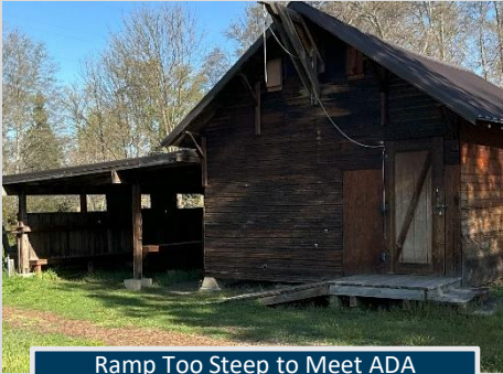
Ramp Too Steep to Meet ADA Requirements
