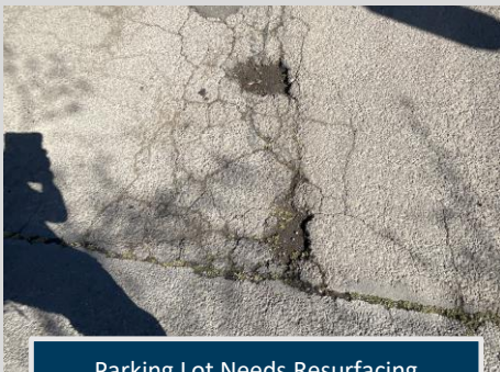
Parking Lot Needs Resurfacing
