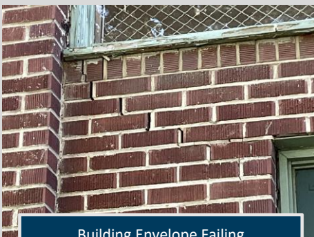
Building Envelope Failing
