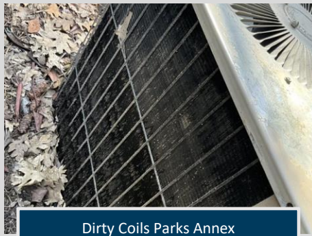
Dirty Coils Parks Annex
