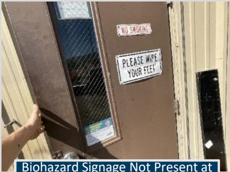
Biohazard Signage Not Present at Welding Shop
