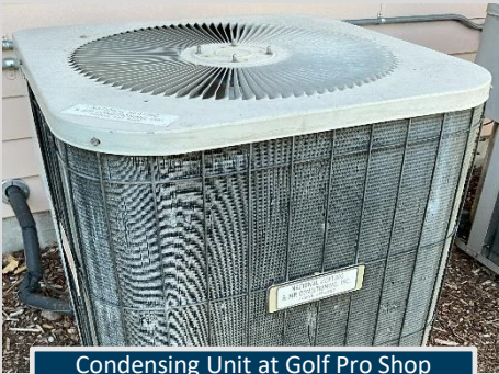
Condensing Unit at Golf Pro Shop Beyond Useful Life Expectancy.
