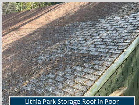
Lithia Park Storage Roof in Poor Condition
