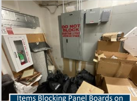
Items Blocking Panel Boards on 2nd Floor
