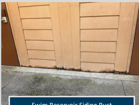
Swim Reservoir Siding Rust
