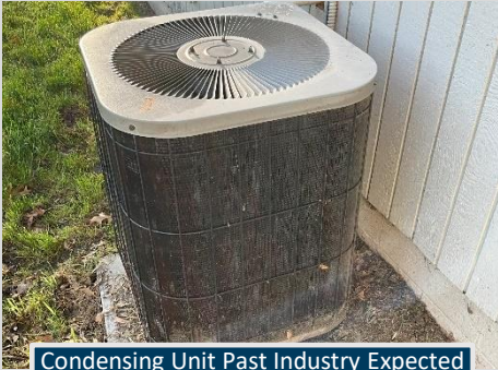
Condensing Unit Past Industry Expected Life
