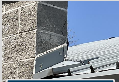
Flashing Needs Replacement
