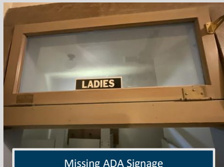
Missing ADA Signage
