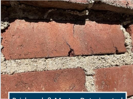
Brickwork & Mortar Deteriorated
