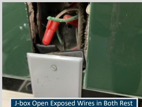
J-box Open Exposed Wires in Both Rest Rooms
