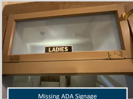
Missing ADA Signage
