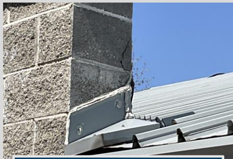
Flashing Needs Replacement
