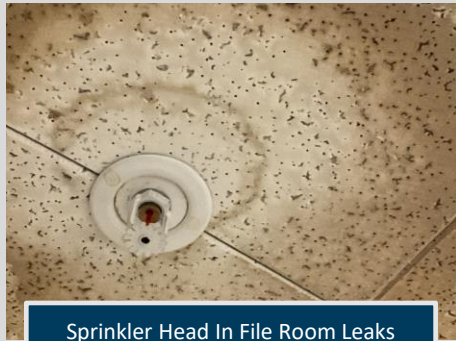
Sprinkler Head In File Room Leaks
