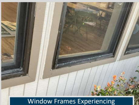
Window Frames Experiencing Weathering
