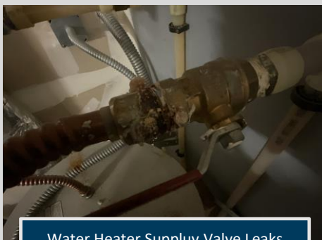
Water Heater Supply Valve Leaks
