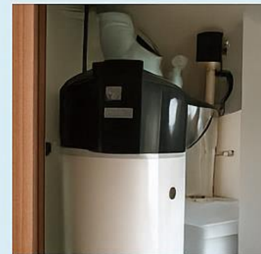
Hot Water Heat Pumps
