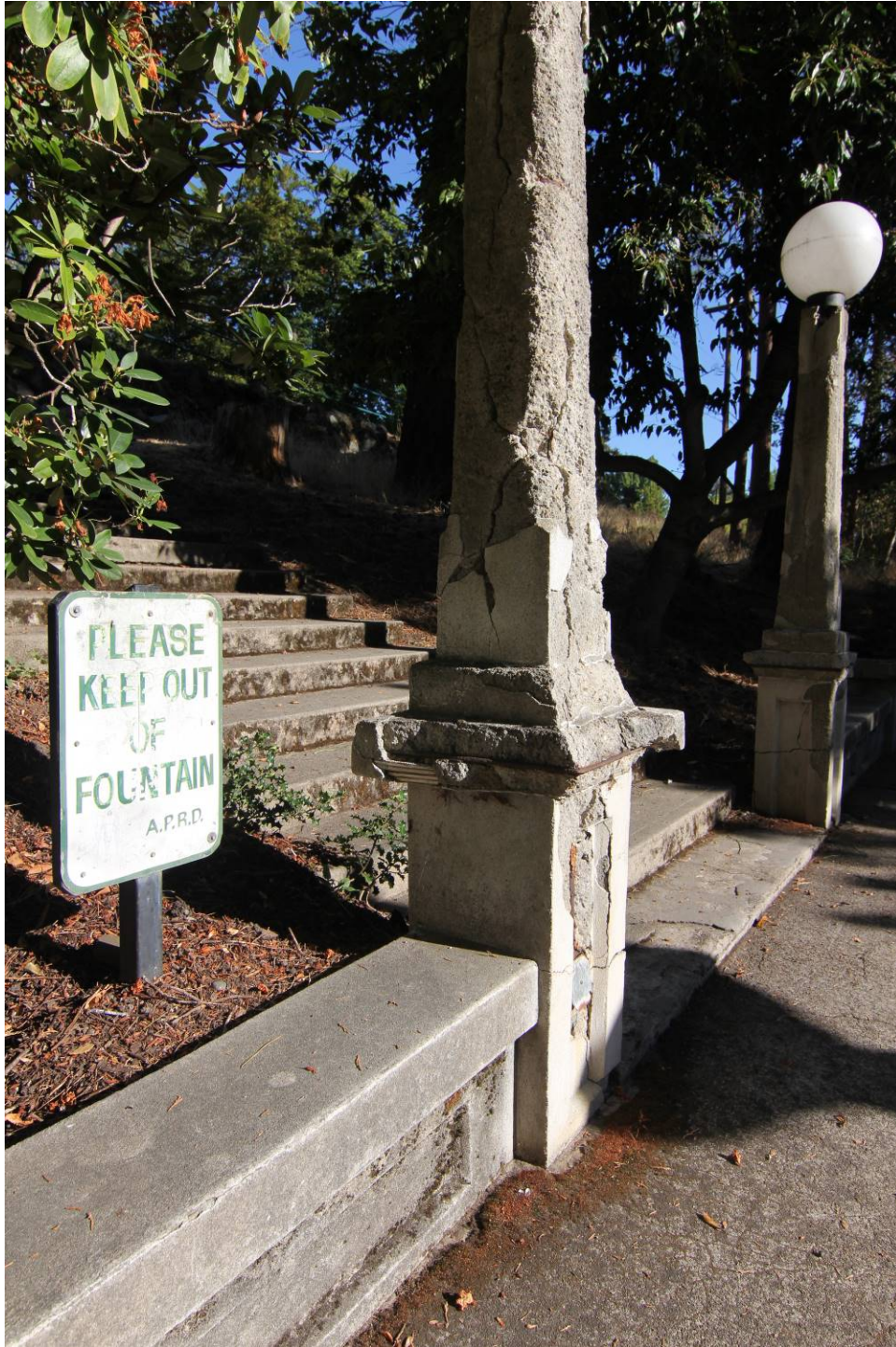
FIGURE 18. CURRENT IMAGE, Light Standard (note damage) G. Kramer Image, 2025
