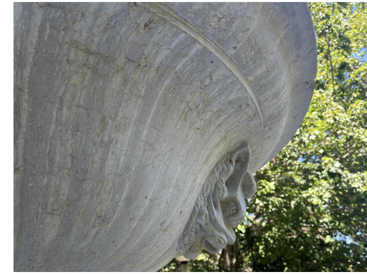
MH-1: MARBLE HAIRLINE CRACK REPAIR CONDITION: CRACK IN MARBLE OF VARIABLE LENGTH UP TO 1/4" IN WIDTH. REPAIR: GROUT TO MATCH EXISTING MARBLE ESTIMATED QUANTITY: ALL HAIRLINE CRACKS AT EXISTING STONE
