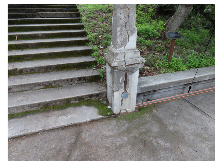
CP-1 CONCRETE PARGE REPAIR PROVIDE CONCRETE PARGE REPAIR AT TERRACE SIDE OF (E) CONCRETE WALL FROM BOTTOM OF WALL PANELS TO TOP OF NEW SLAB (T.O. NEW SLAB WILL BE BELOW THE T.O. (E) TOPPING)
