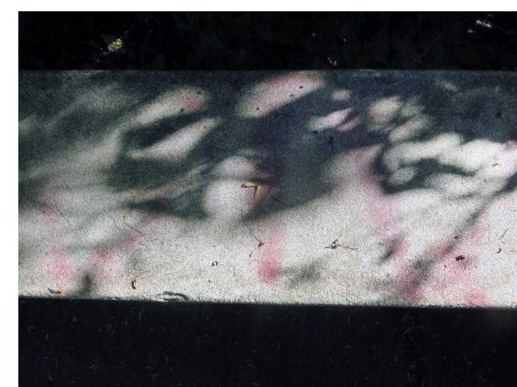
CG-1: CONCRETE GRAFFITI CLEANING CONDITION: LOCALIZED MODERATE TO HEAVY SOILING THAT COMPRISES MATERIAL REQUIRING SPECIALIZED REMOVAL SUCH AS GRAFFITI REPAIR: CLEAN CONCRETE TO REMOVE GRAFFITI ESTIMATED QUANTITY: 20 SQUARE FEET
