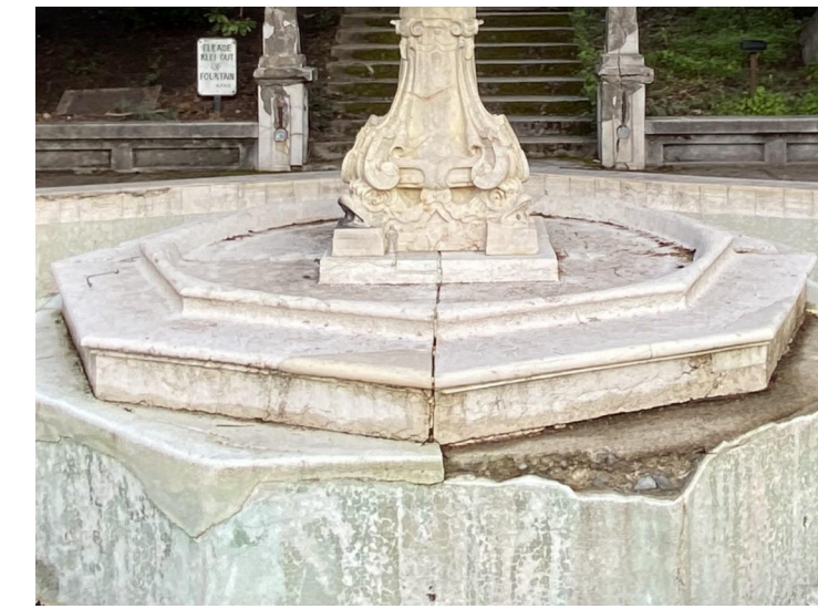
MARBLE FOUNTAIN STEPPED STONE BASE & POOL REPLACE MARBLE STEPPED STONE BASE & POOL WITH MARBLE TO MATCH EXISTING
