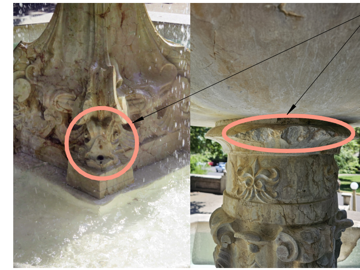
MS-1: MARBLE SPALL REPAIR CONDITION: SPALL AT SURFACE OF MARBLE REPAIR: PROVIDE PROFILED MARBLE DUTCHMAN REPAIR ESTIMATED QUANTITY: 7 LOCATIONS
