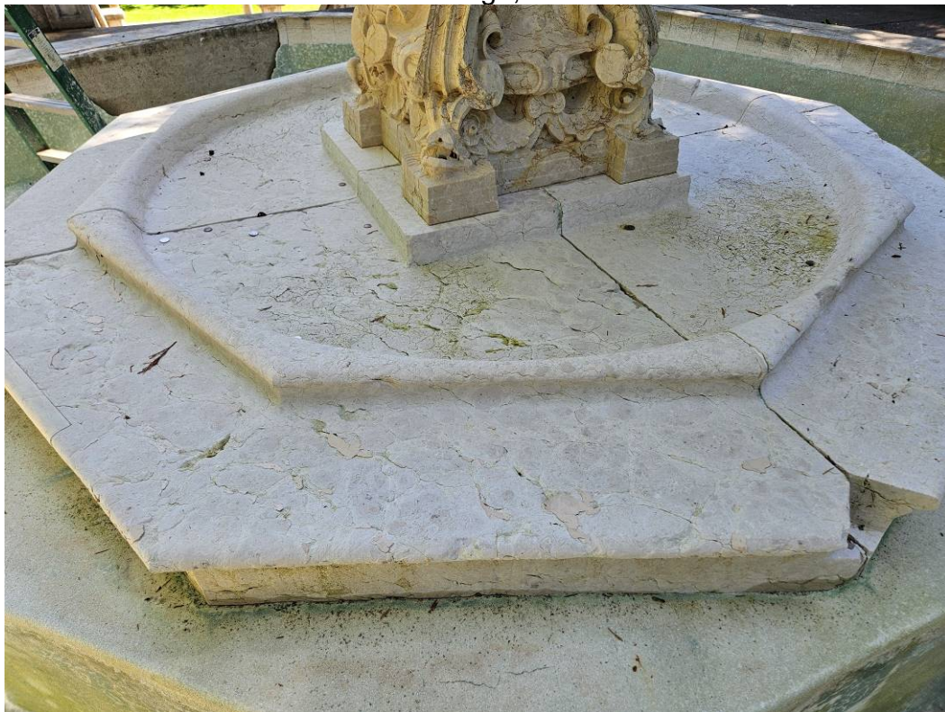
FIGURE 20. CURRENT IMAGE, Lower Pool, Marble Damage ARG Image 2025
