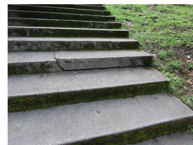
CONCRETE STAIR DISPLACEMENT GRIND DOWN DISPLACED AREA, & PROVIDE CRACK FILL REPAIR
