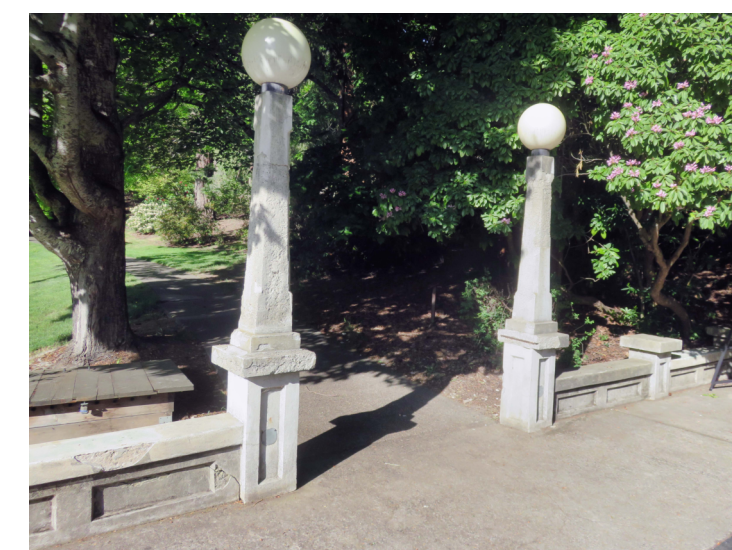
CONCRETE LIGHT STANDARDS REPLACE WITH PRECAST CONCRETE LIGHT STANDARDS TO MATCH EXISTING
