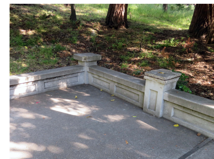
CONCRETE (TO REMAIN), INCLUDING CHEEKWALLS, PIERS, WALLS, UPPER STAIR, AND LOWER STAIR 100 PERCENT OVERALL CLEANING OF EXISTING CONCRETE TO REMAIN
