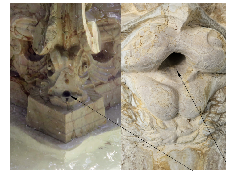
MD-1: MARBLE DRAIN OUTLET REPAIR REPAIR: CLEAN OUT EXISTING DRAINAGE FROM BOWL TO OUTLET. IMPROVE BORE & POLISH OUTLET AS NEEDED TO CREATE LAMINAR FLOW OF WATER ESTIMATED QUANTITY: 4 LOCATIONS AT BASE, AND 4 LOCATIONS AT LOWER BOWL DRAIN OUTLET AT LOWER BOWL DRAIN OUTLET AT BASE OF PEDESTAL; LOCATION ALSO SHOWS MS-1 REPAIR TYPE
