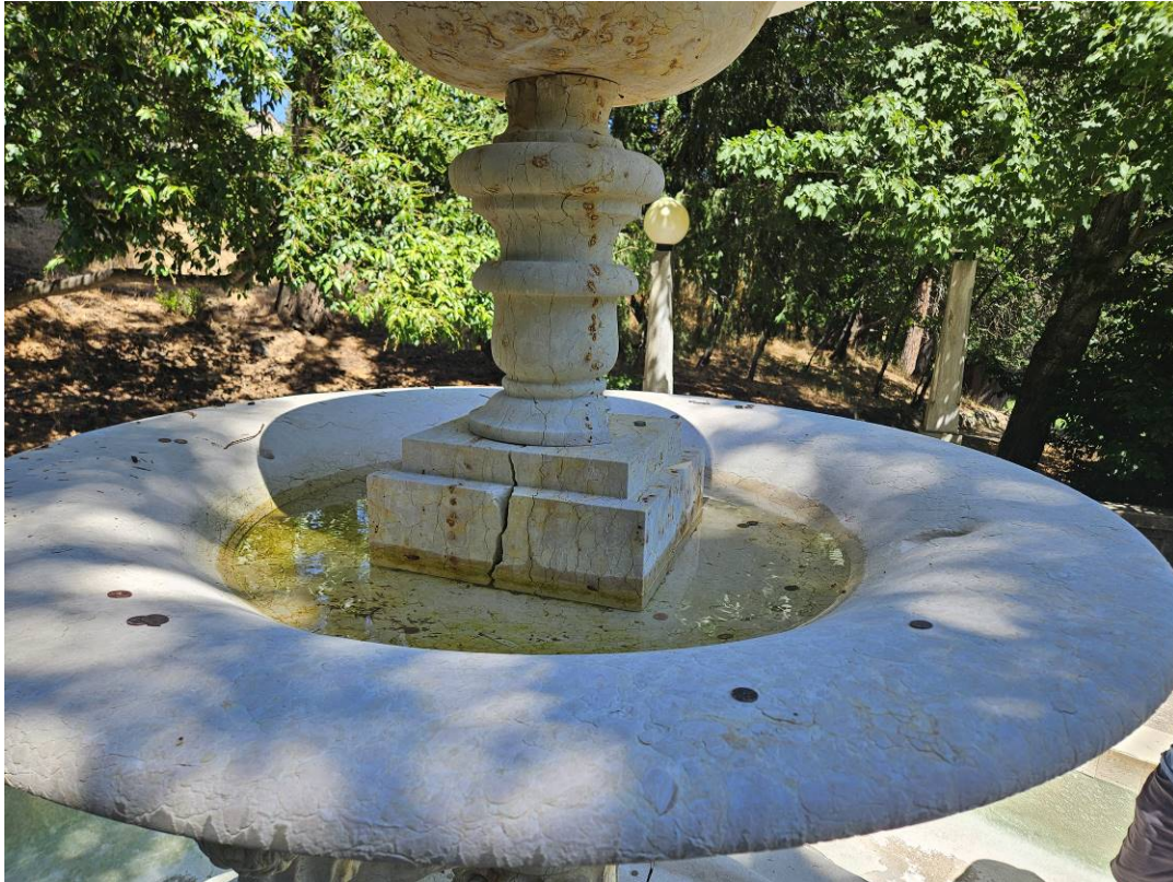
FIGURE 19. CURRENT IMAGE, Middle Pedestal Damage ARG Image, 2025
