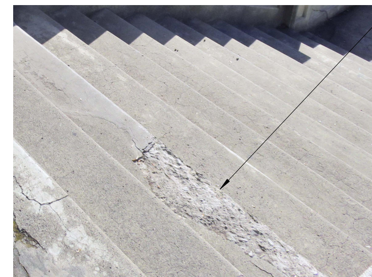
CS-1: CONCRETE SPALL REPAIR CONDITION: SPALL AT CONCRETE, SURFACE AREA VARIES REPAIR: PROVIDE CONCRETE PATCH REPAIR ESTIMATED QUANTITY: 52 SQUARE FEET, 34 LOCATIONS
