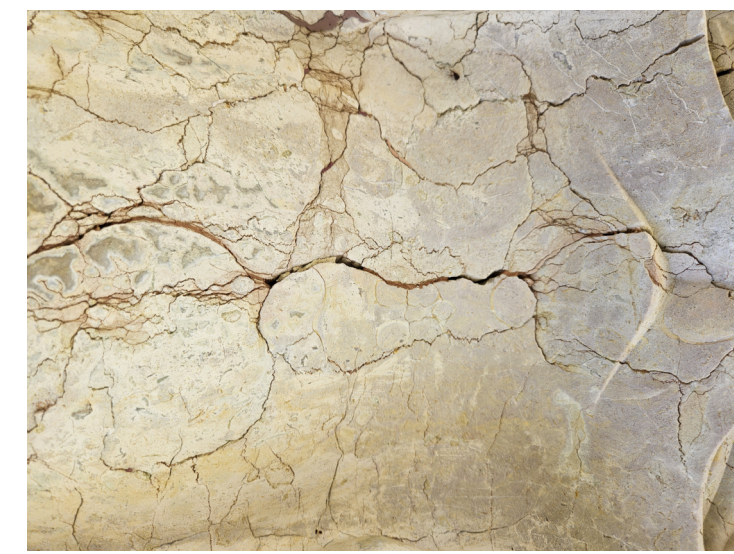
MC-1: MARBLE CRACK REPAIR CONDITION: CRACK IN MARBLE OF VARIABLE LENGTH GREATER THAN 1/4" IN WIDTH. REPAIR: PROVIDE CRACK FILL REPAIR ESTIMATED QUANTITY: 4 LINEAR FEET
