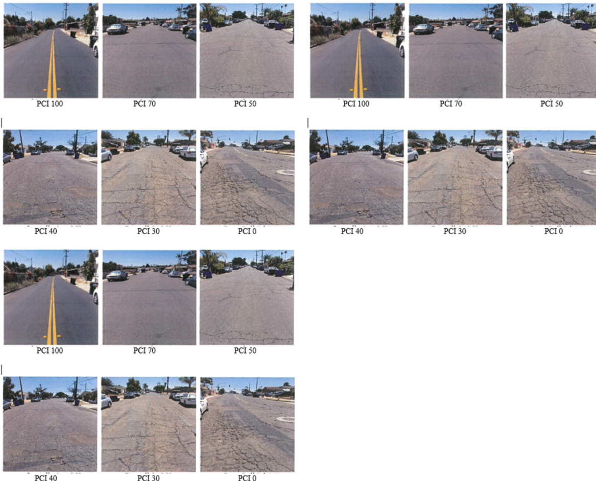
Figure 1: Pavement Condition Index
